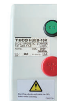
Motor ON/OFF switch box
